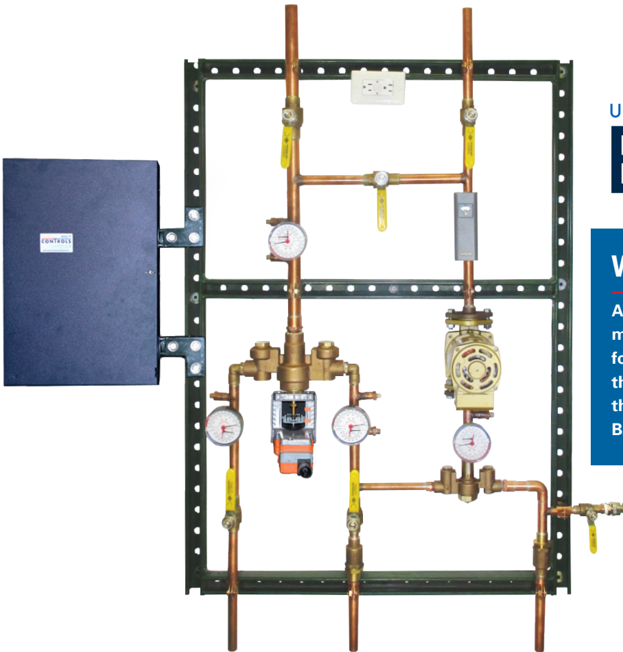
COMMAND STATION UPGRADED WITH BASyC
